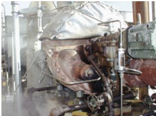
FIG. 2 Pure oil mist installation on a steam turbine.
