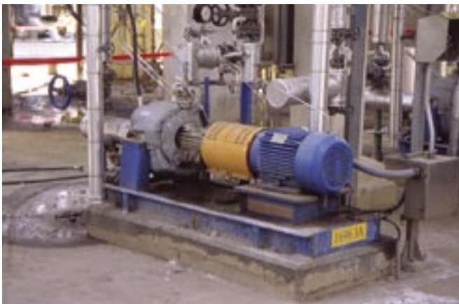
FIG. 1 Pure oil mist installation on a pump and motor (API 610 application).
